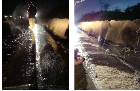
Figure 2: Leaking after conventional crack sealing
