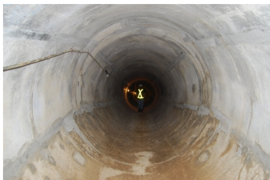
Figure 4: Initial interior surface conditions of the pipeline
