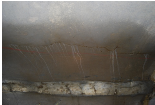
Figure 3: Seepage water draining into pipeline
