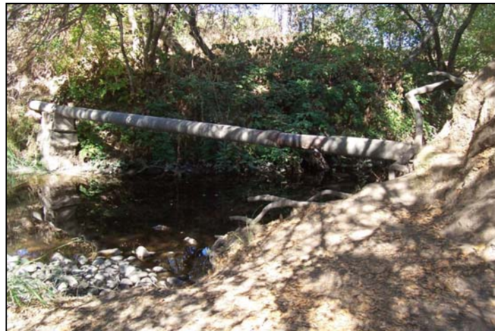
Photo 3 – A structural engineer performed field visits to sites where potential structural deficiencies were identified during the initial field visit.
