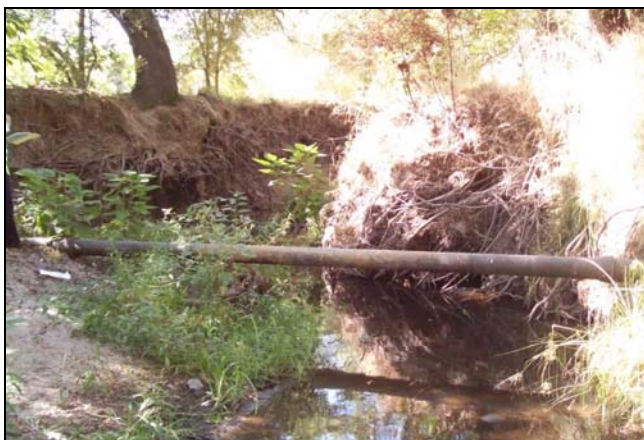
Photo 1 – Site 13 consists of a cast iron pipe that was originally buried and was exposed as the creek incised over time.
