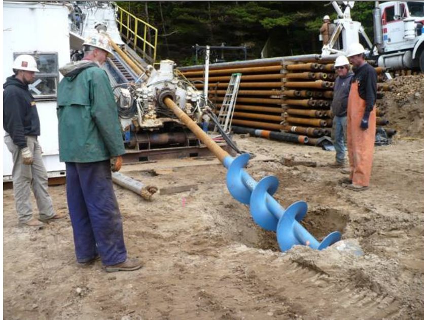
Figure 5. Photograph of auger flight used to remove spoil from inside conductor casing
