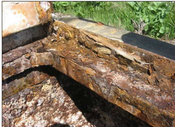
Figure 2. Corroded Frame of JB 68-9
