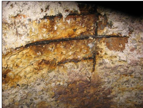
Figure 3. Exposed corroded reinforcing steel MH 79-13
