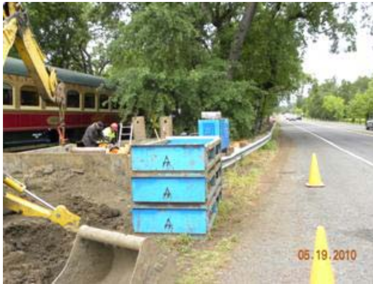
Figure 1. Tight conditions. Note: A State highway on one side of the jobsite and a rail line on the other.
